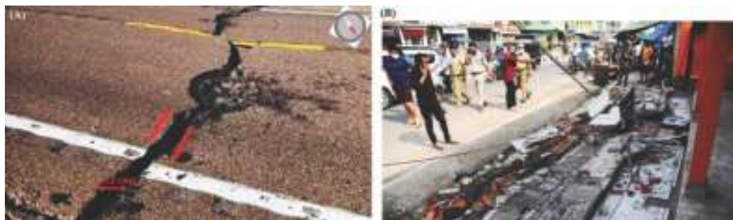
Fig. 2. Example of fractures and cracks occurring in many places around the Dhekiajuli region. The falling of bricks walls in the Dhekiajuli is shown in image B, collecting from Press Trust of India (PTI, 29 April, 2021).
