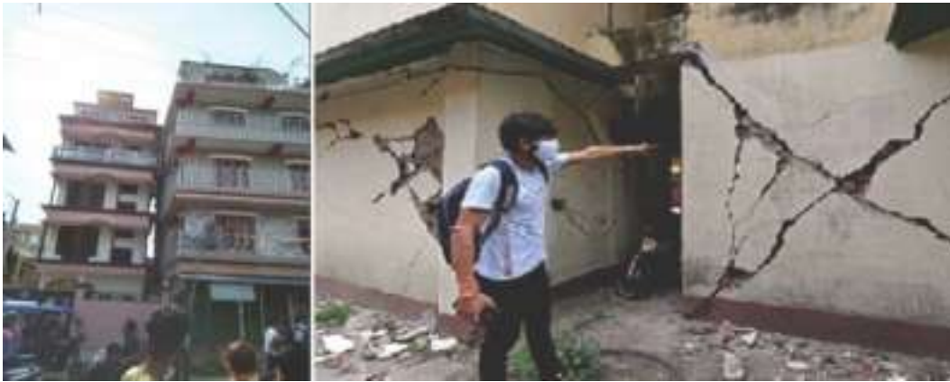
Suppl. Fig. S2. Damage scenario in residential constructions at Tezpur town, nearly 30 km away from epicenter of the mainshock.
